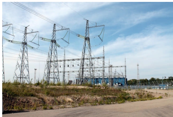
Photo 5.6: High Voltage Power Lines
